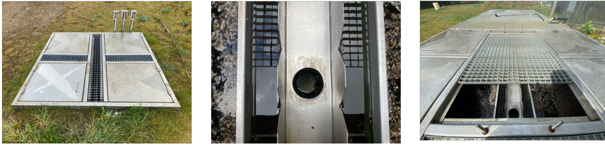
Figure 10: Pictures of biological wastewater treatment plant BIO M-30 (photos: Zviedris J., VNK serviss Ltd.).
