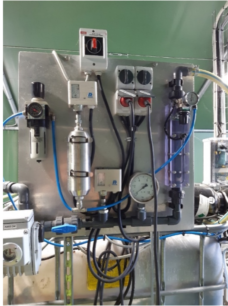
Figure 4: External nano bubble generator (Anzii unit) installed to produce nano bubbles, the unit have been connected to water pump and air supply (photo: Morten Lykkegaard Christensen).
