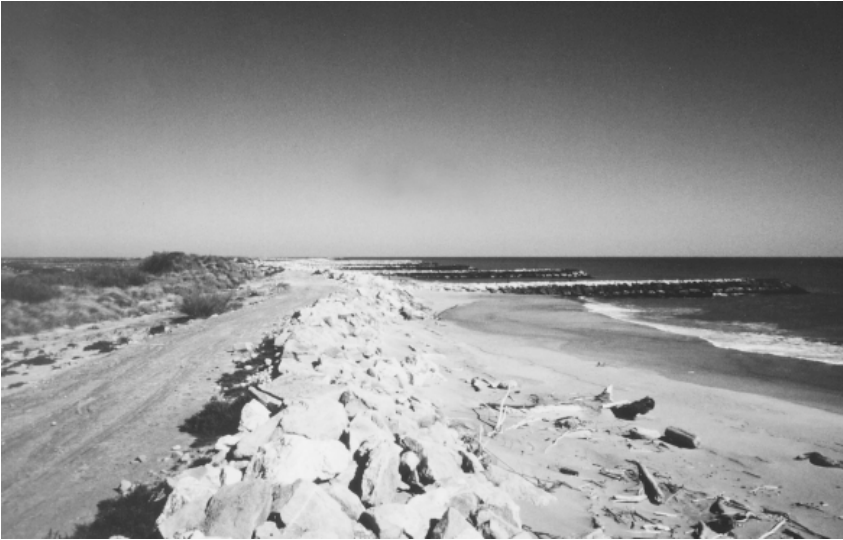
Fig. 3. Frontal dike and groynes established on the littoral of Faraman (la Galère lagoon area).
