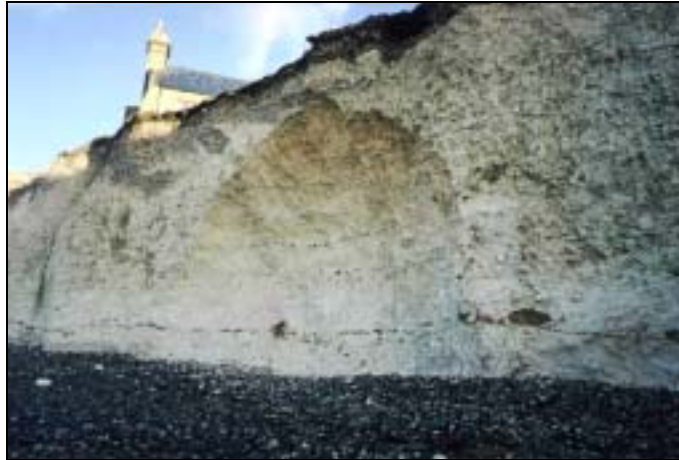
Fig. 12: Threatened building at Birling Gap.
