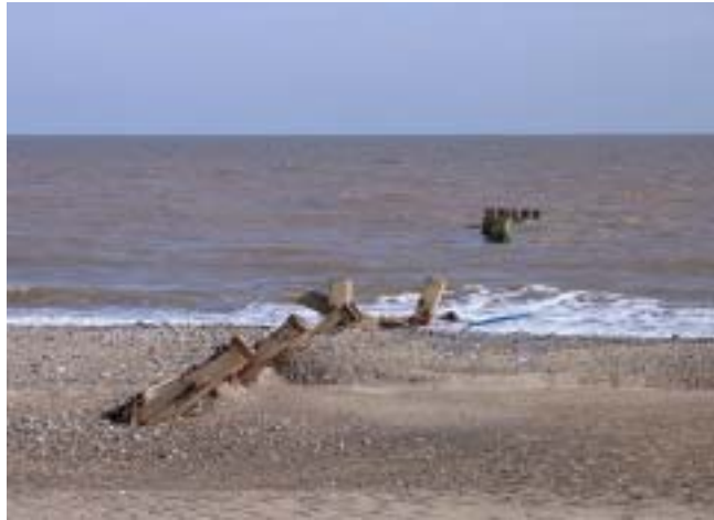
Fig. 05: Timber groin, destroyed by lowering of the beach.
