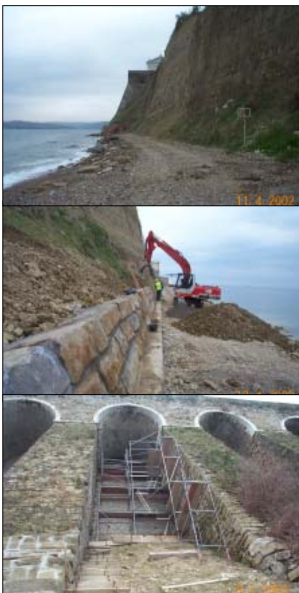
Figs. 16,17,18: Recent erosion protection works in the historic town of Piran. (Source: Archive of Podjetje za urejanje hudournikov, Ljubljana).
